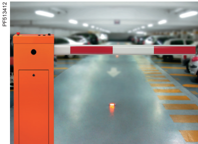
ATV12 controlling an access barrier
